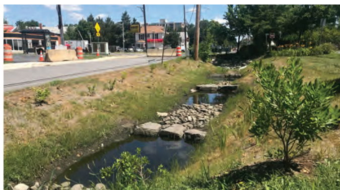
Example of a sloped swale and rain garden using large stone buffers as check dams to reduce runoff velocity and allow for infiltration. Fig. 089b | (SMC, 2015)
